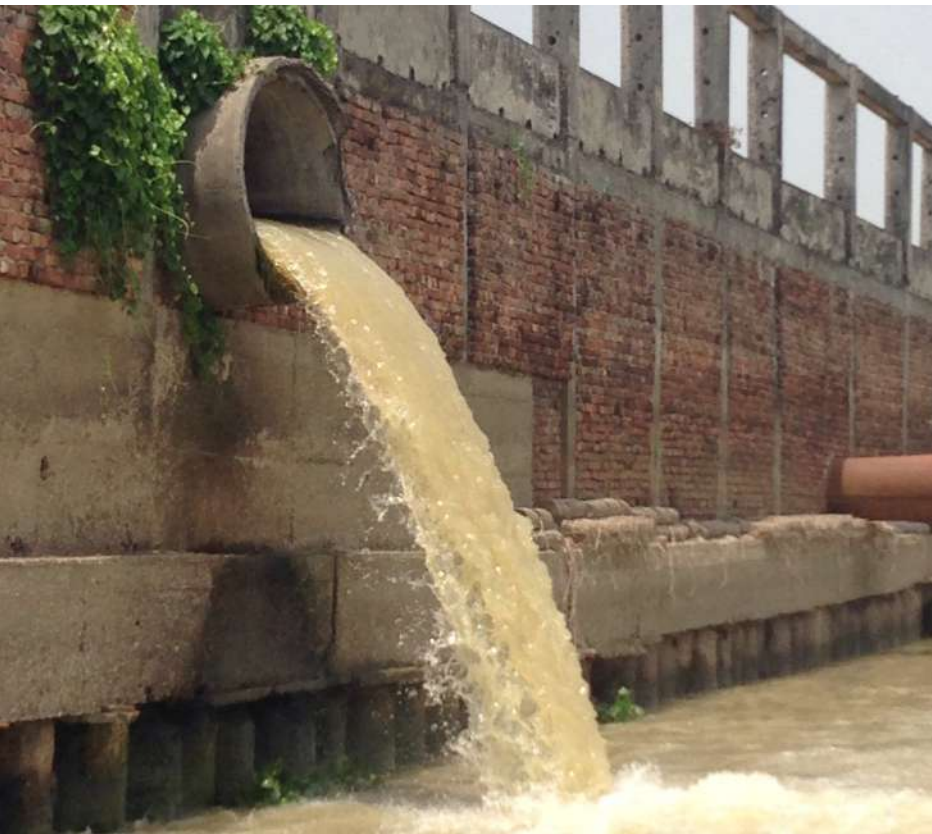
Direct industrial outfall into the Meghna River at the west bank near Meghna Bridge
