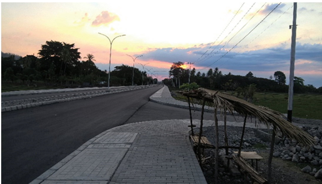
Pante Macassar Street. Newly constructed urban street in the city of Pante Macassar (photo by Robert Haywood).
