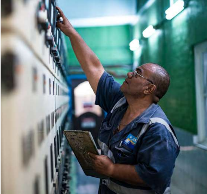
A worker monitors power loads at the Nauru Utilities Corporation. ADB has helped residents of the island nation enjoy access to cheaper, cleaner, and more reliable electricity.
