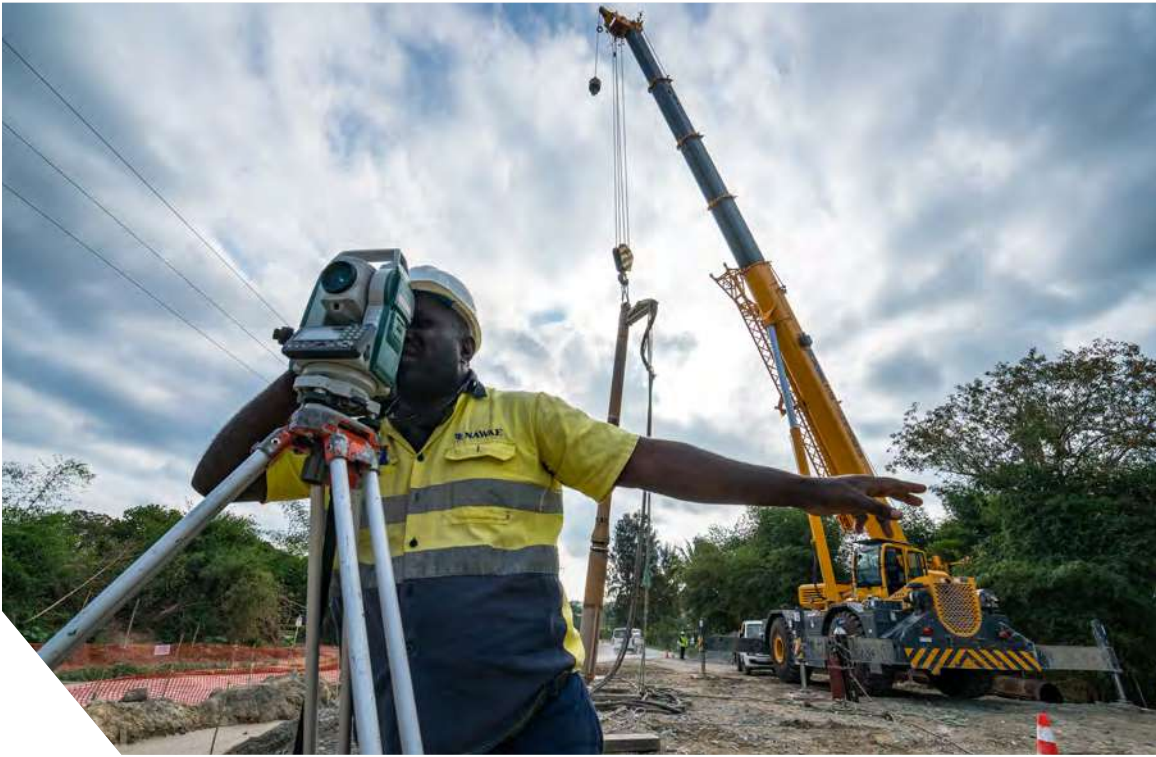
ADB is rebuilding roads in Vanuatu to standards that make them climate and disaster-proof. Under Strategy 2030, ADB is stepping up its support to address climate change, disaster risks, and environmental degradation, especially in vulnerable countries.
