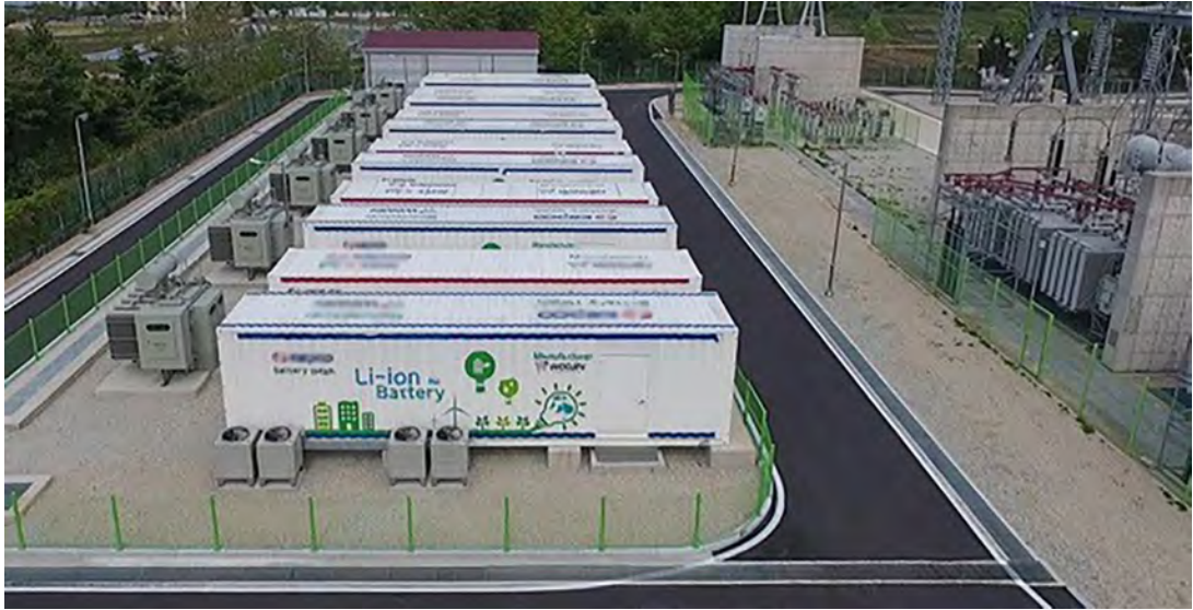
Figure D.4: Sokcho Battery Energy Storage System
