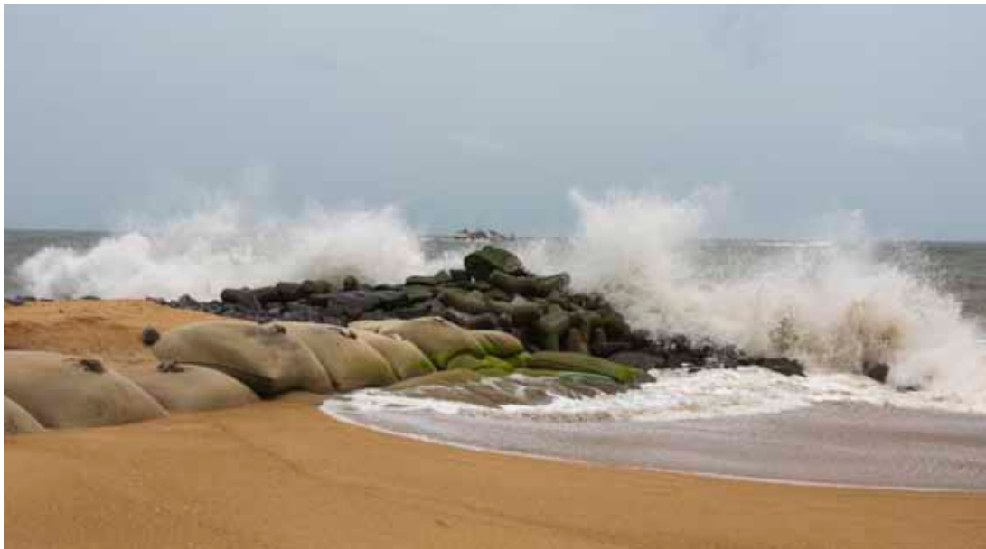
Beach protection. Construction of berms under the Sustainable Coastal Protection and Management Investment Program, Ullal, Karnataka, has reclaimed the beach and protected the assets of fishing communities (photo by ADB).
