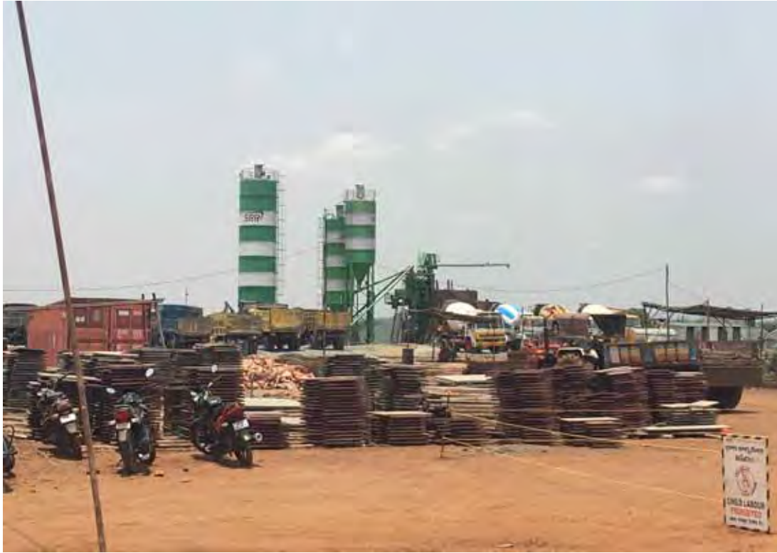
Corridor development. Ongoing infrastructure development at Naidupeta Cluster under VCIC in Andhra Pradesh (photo by ADB).
