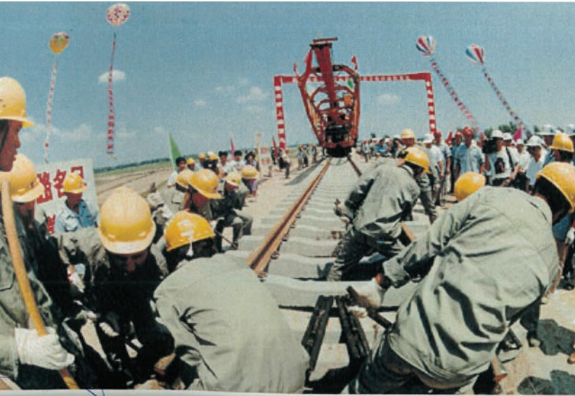
The Jing-Jiu Railway Technical Enhancement Project was approved in 1994. The project installed high-quality rails on a 600-kilometer section of the Jing-Jiu railway, doubling its capacity and improving efficiency and safety.
