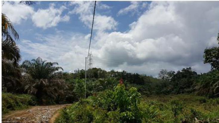
Low Voltage (LV) lines along access road to households
