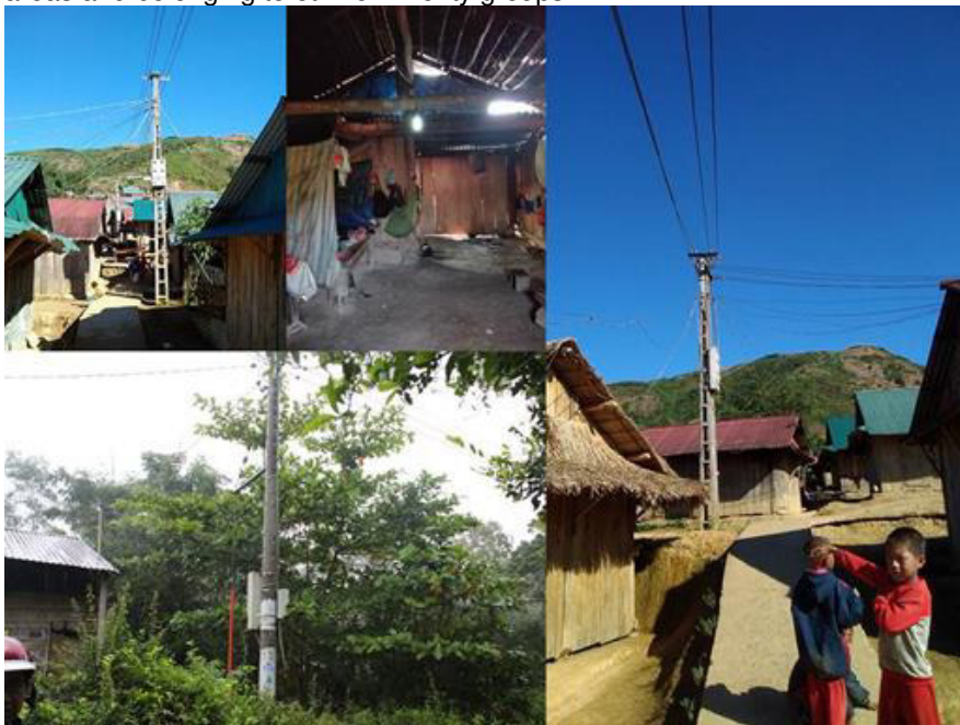
Low Voltage Line along Commune Road and Service Connections; and Service Connection from Power Meter to the House
