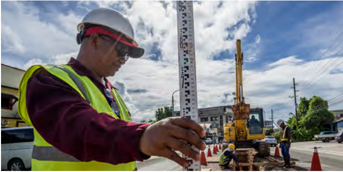
Sewerage system construction in Koror, Palau. The Koror-Airai Sanitation Project aims to improve sanitation services in Airai and Koror, where about 80% of the country's population live.
