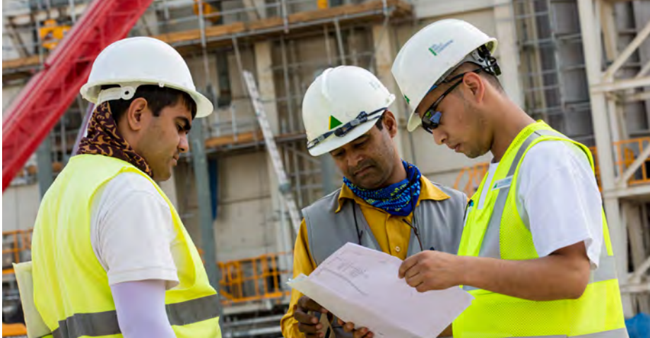
Engineers confer on construction works for the Talimarjan Power Plant in Uzbekistan. Built with ADB support, this 800-megawatt gas plant will boost the country's energy efficiency.
