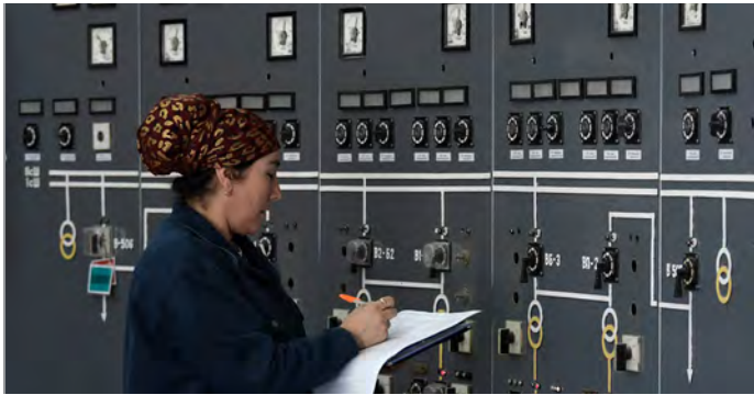
A duty electrician collects energy data at the Nurek Hydropower Plant in Tajikistan. ADB provided $55 million to reconstruct the switchyard at the plant, which produces over 70% of Tajikistan's electricity.
