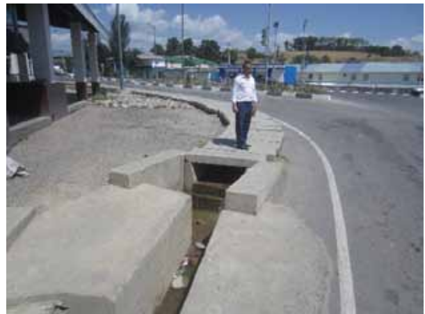
Being able to identify a roadside hazard, and then knowing what are the best options to treat the hazard, is an important job for highway engineers.
