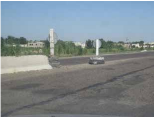
Old tires and similar untested and nonapproved devices must not be used to shield the ends of rigid or semirigid barriers.
