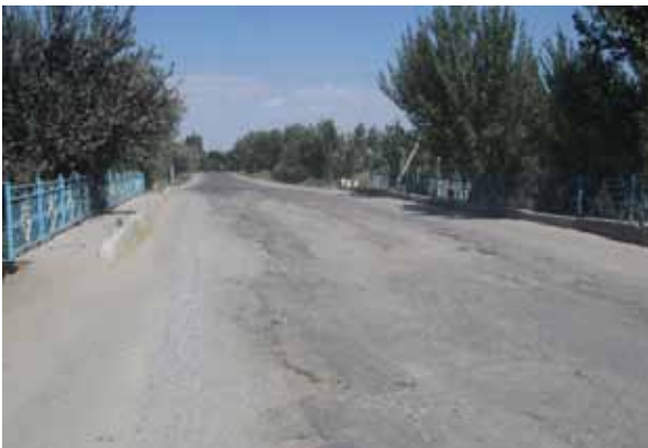
There are three small bridges (like this), a larger bridge, and 20 culverts in the 55-kilometer length to be rehabilitated.
