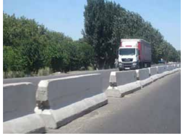
Individual concrete barricades like these may be able to prevent illegal turns, but they are hazardous, especially if struck on their exposed ends.
