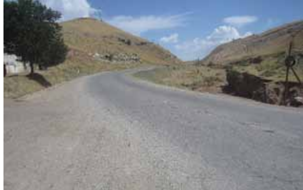
Operating speeds are around 80 kilometers per hour. Volumes are almost 4,000 vehicles per day (total both directions). The highway lacks delineation. Many of the single-vehicle crashes occurred at night.
