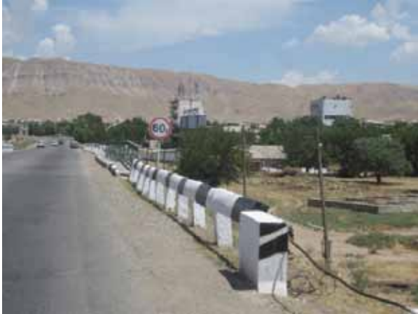
Concrete blocks and concrete barriers like these are roadside hazards. At best, they offer limited delineation only.
