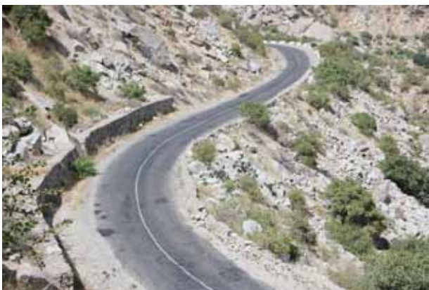
The highway is a two-lane, two-way highway passing through hilly terrain. It has generous geometry but it has numerous roadside hazards along its length.
