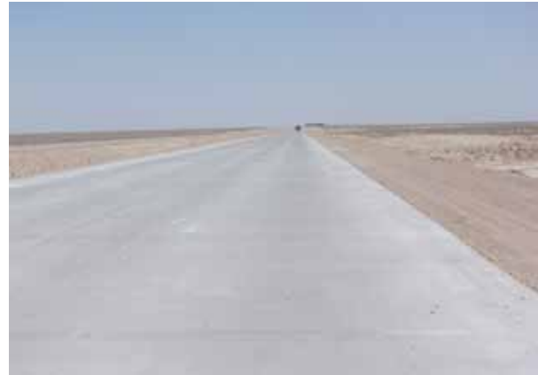
The pavement encourages high speeds, but there is little to assist, guide, inform, warn, or control drivers.
