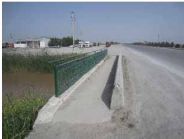
Bridge railings must be strong enough to contain an impacting vehicle. Light gauge rails, such as this, are not strong enough for this task. The low concrete barrier is another hazard.
