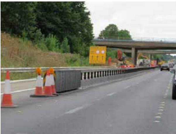
Some impact attenuators are designed to be used in narrow areas at road work sites.
