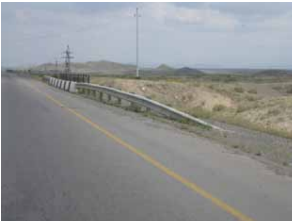
Ramped terminals, such as this, are not to be used on high-speed sections of CAREC highways, except on the trailing end of barrier on one-way carriageways.
