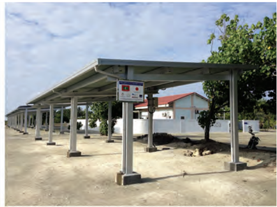
Shade structure ground-mounted—Dhiffushi, Maldives
