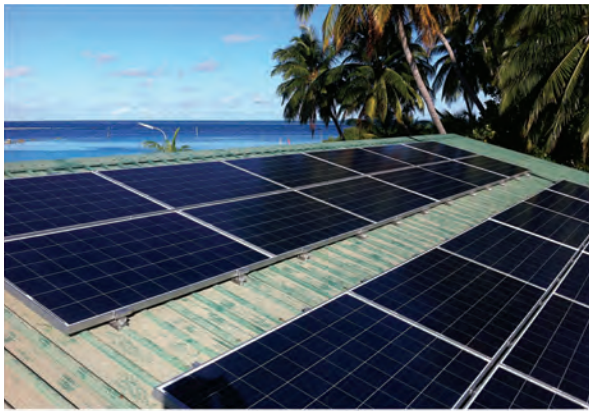
Rooftop mounted—Dhidhdhoo, Maldives
