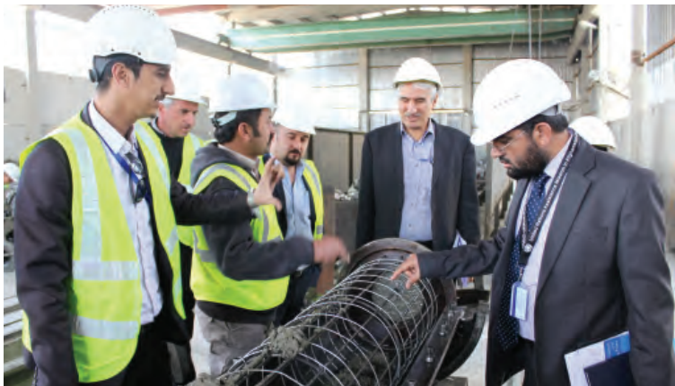
Hamidullah Durrani ( right ) of the Afghanistan Resident Mission visits a concrete pole factory in Kabul. ADB's reengagement with Afghanistan began in 2002.
