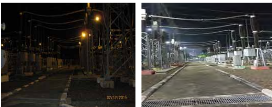
Figure E1: Lighting Conditions at Cilegon Substation Before and After the LED Retrofit
